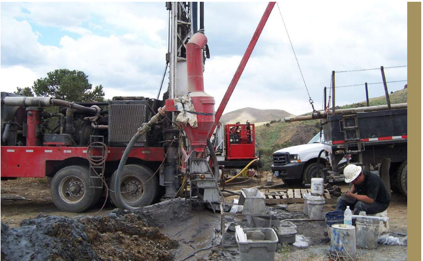
Drilling by JV partner Platte River at Chert Cliff gold project, Nevada
